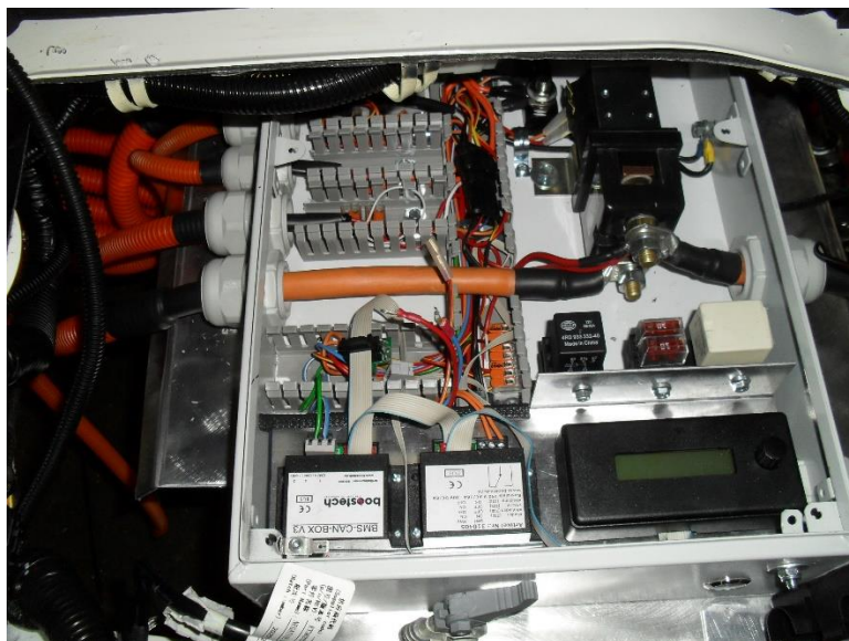
Hauptstromkasten mit: 1. BMS-Master Unit, 2.CAN BUS Relais,
